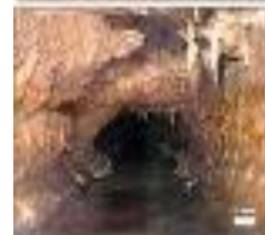
Grease filled sewer line
