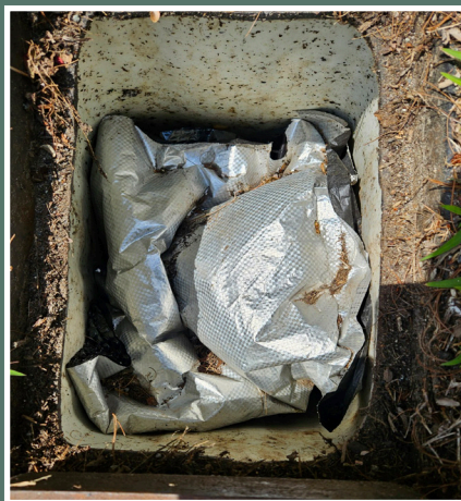
New meter with meter blanket
