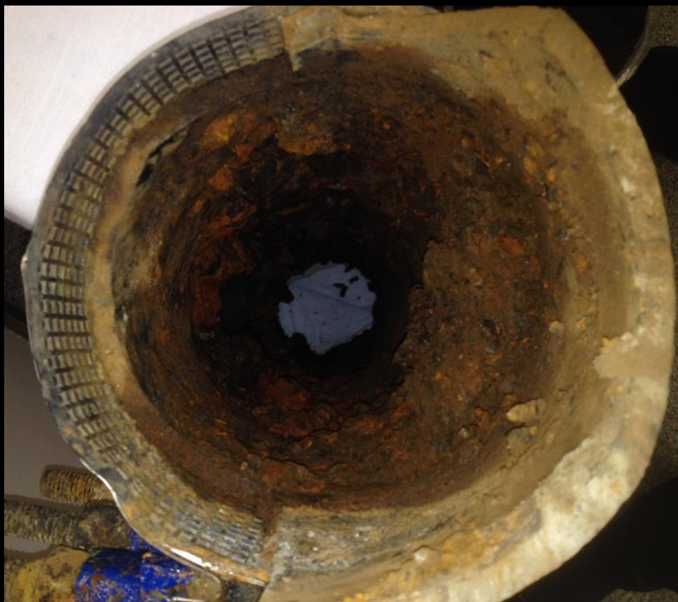
6" Cast Iron Pipe
