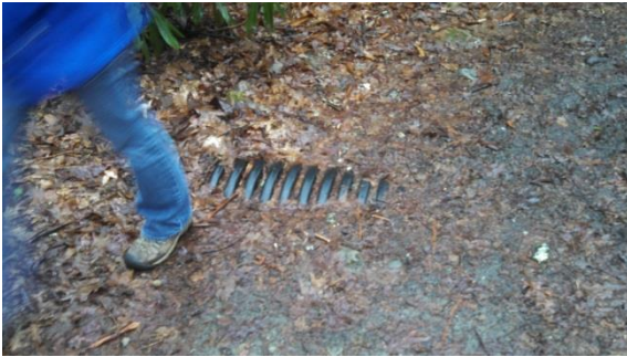
Example 1 – Failing culvert
