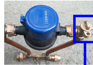
Water meter shut off valve
